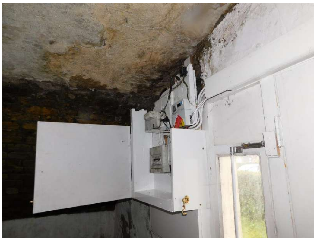
Photograph 1 – water entry above fuse box
