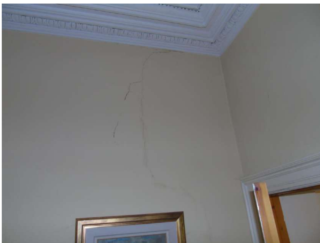
Photograph 6 – Plaster damage and water infiltration adjacent to room door.
