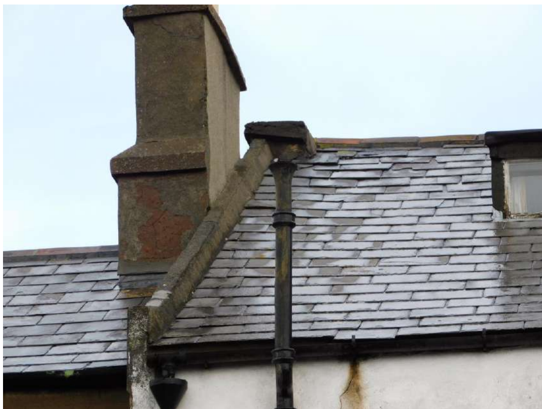
Photograph 3 – sagging roof/missing and damaged tiles/dilapidated dormer window projections.
