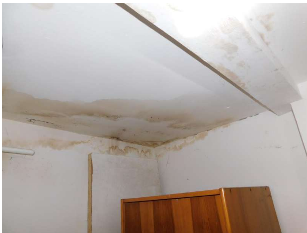
Photograph 2 – flat roof breached by rainwater
