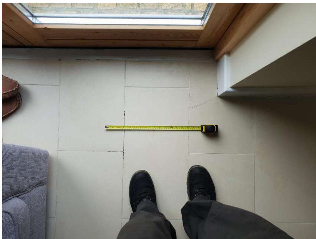
Photograph 5 – possible pyrite related floor tile cracking and grout loss.
