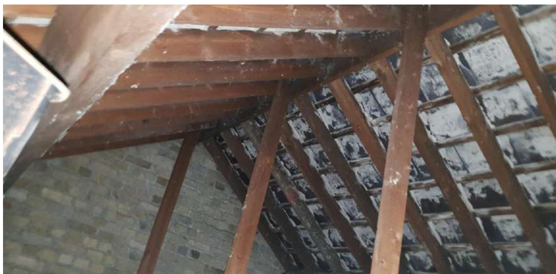
Photograph 4 – failing lime torching to underside of roof tiles.
