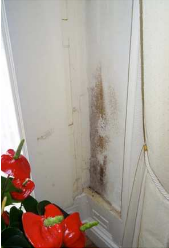
Figure 17: Mould growing behind shutters
