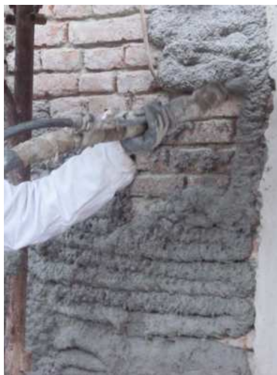
Figure 59: Insulating render spray applied on external walls. Spraying can use less material than application by trowel because the plaster is not being compacted.
