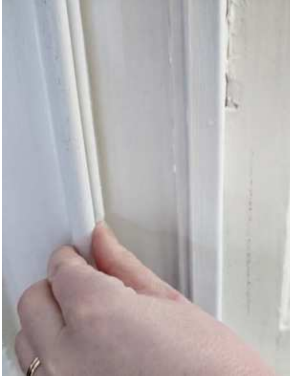
Figure 49: Discreet draught-proofing brush on a historic window
