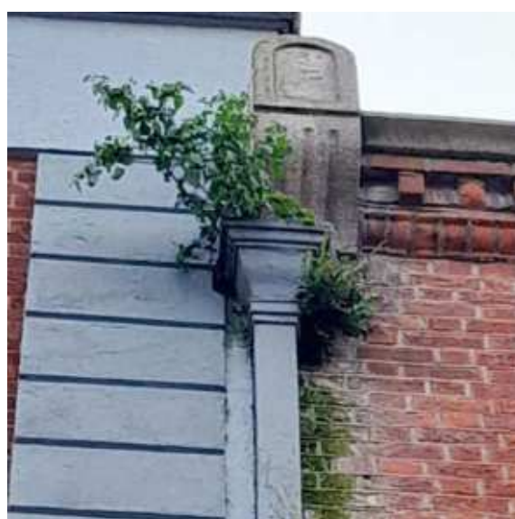
Figure 22: Vegetation growing in a blocked hopper and downpipe
