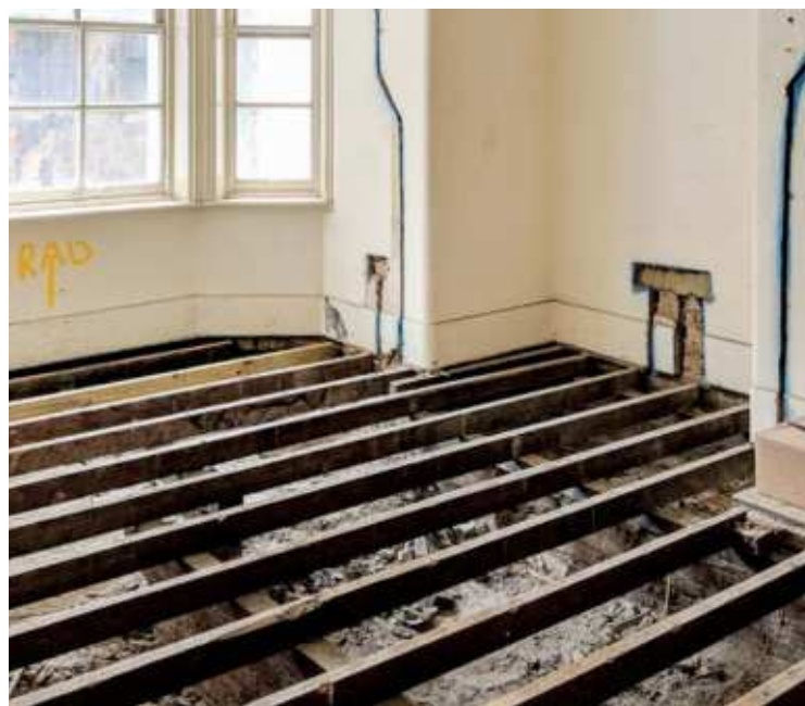
Figure 39: Existing ground floor joists exposed and readied for insulation. The solum should be left free of debris
