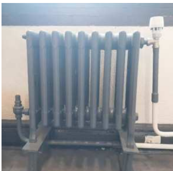
Figure 23: Cast-iron radiator with a thermostatic control
