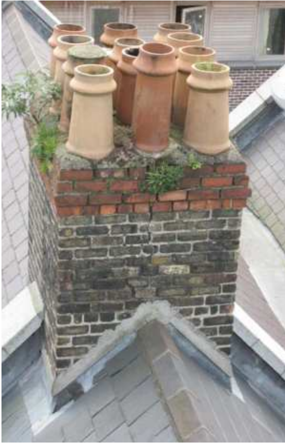
Figure 35: Traditional chimney stack requiring repair and maintenance
