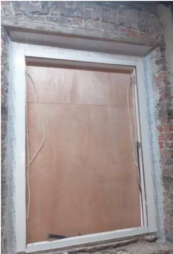
Figure 50: Tape to sash frame prior to application of IWI to ensure an airtight fit (Photograph by Con Brogan for OPW)
