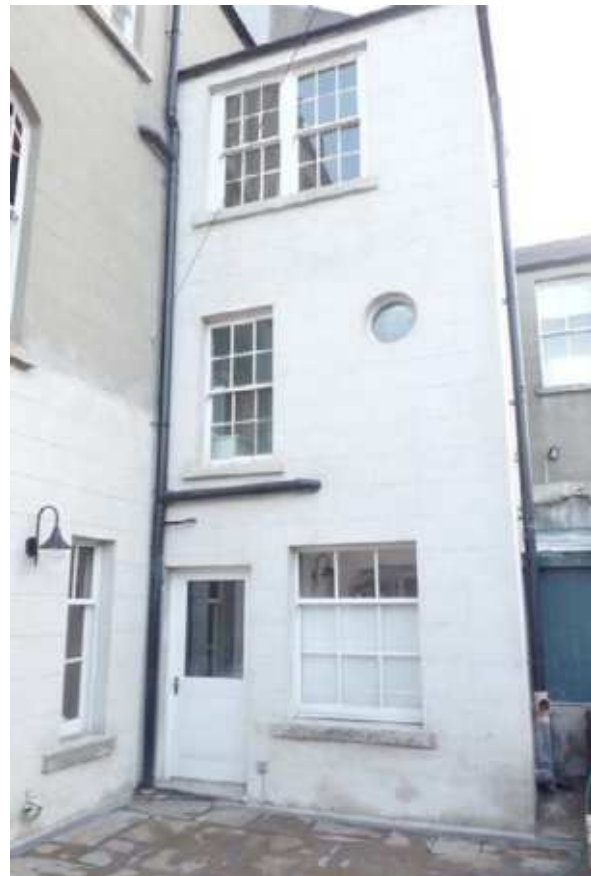
Figure 25: The same building with drainpipe leak fixed and the cement render replaced with a traditional moisture-permeable lime render. Note the addition of a channel drain, which helps to lower the ground moisture level close to the wall
