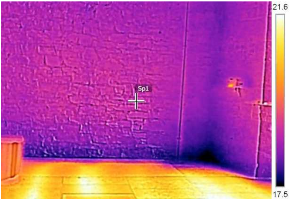
Figure 10: Thermal image showing additional heat flow at vertical and horizontal junctions with the abutting walls and floor. Note that the corner is the coldest point because it loses heat in three dimensions
